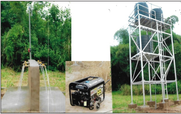
BOREHOLE WITH GENERATING SET AT AGBANIKAKA COMMUNITY, OVIA
