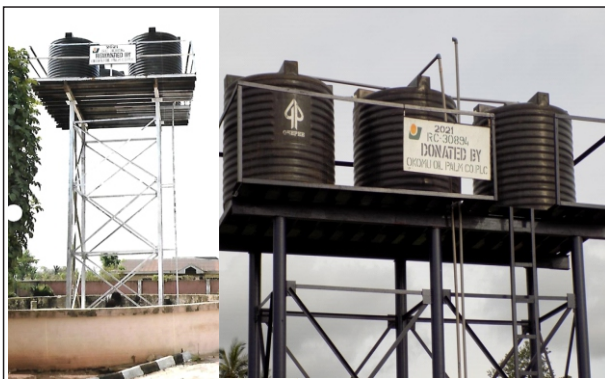
SEMI-INDUSTRIAL BOREHOLE AT THE PALACE OF THE IYASE OF UDO, OVIA SOUTH WEST LOCAL GOVERNMENT AREA & SEMI-INDUSTRIAL BOREHOLE AT MARIOGHIONBA (AT&P) COMMUNITY, OVIA SOUTH WEST LGA CONSTRUCTED BY OOPC
